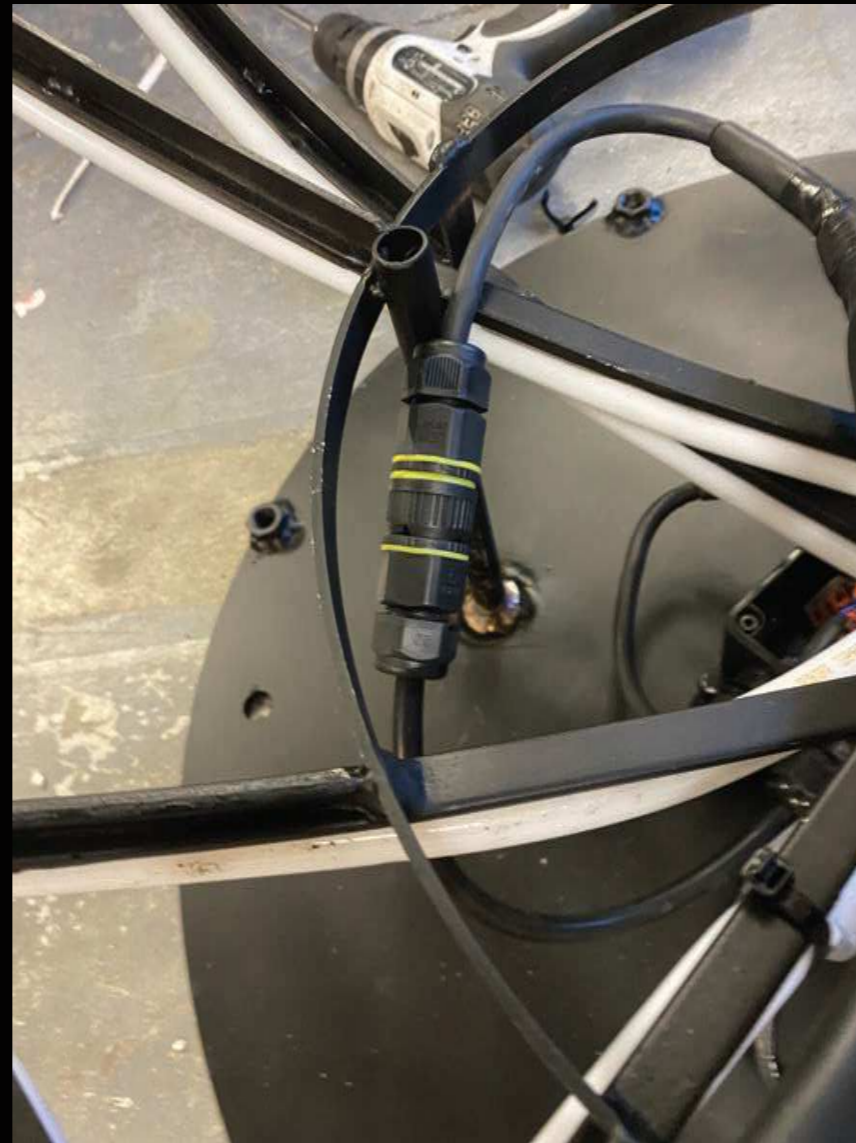
50 m Trailing Yarn IP connection point
